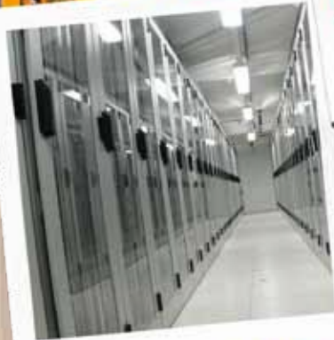
Data centers & UPS systems
